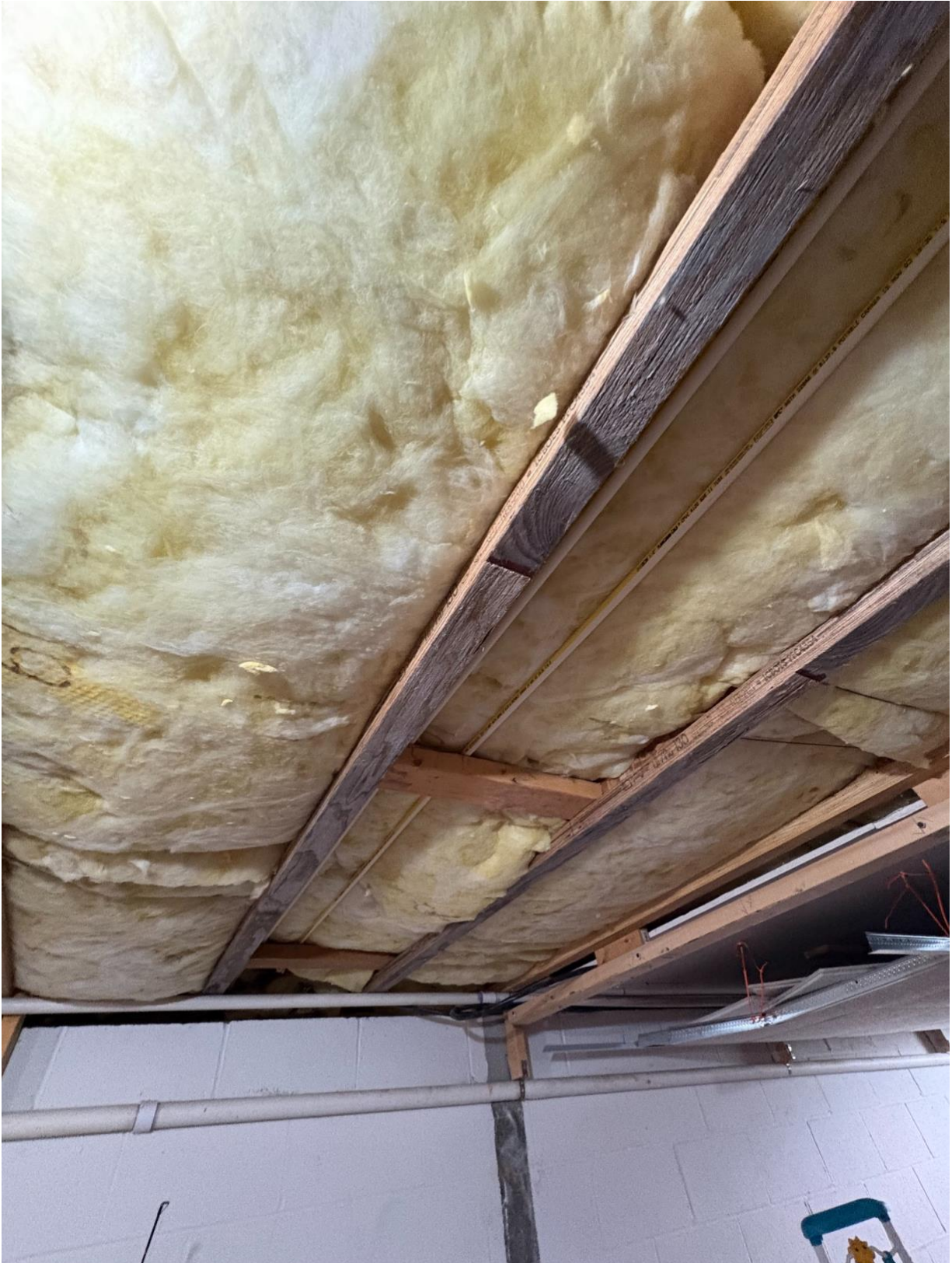
Photo 2 - Example closer view of darker/chalky surface condition along accessible basement joist bottoms.
